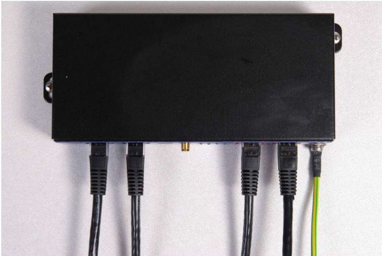
Figure 113 PTP-SYNC mounted on a wall
