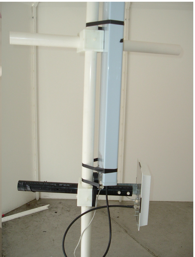
17 dBi cable lay
