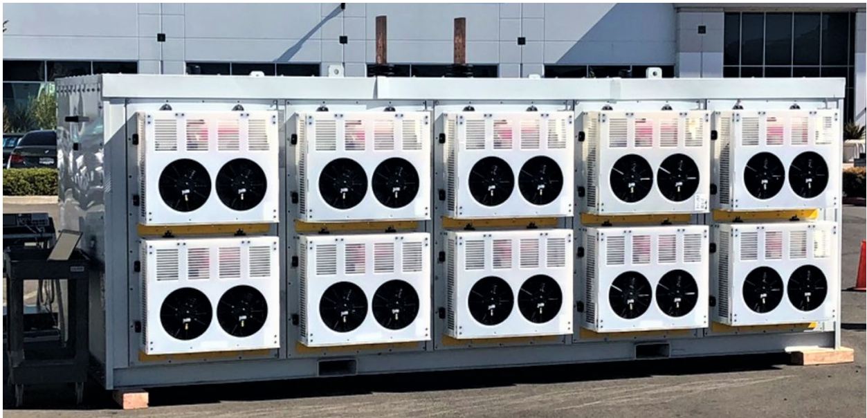
LCS side system view 2
