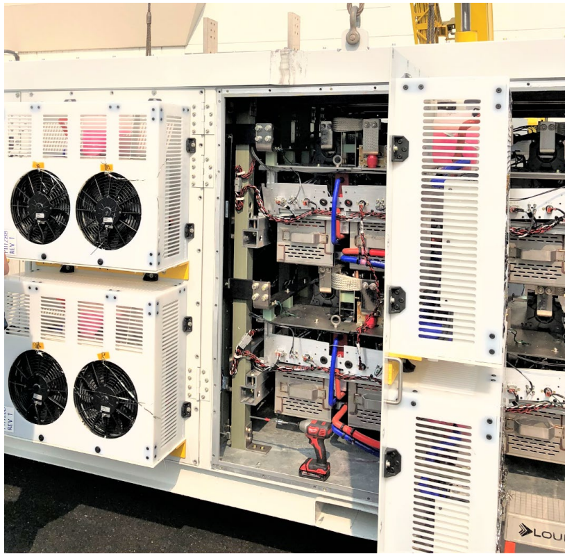
LCS side internal view
