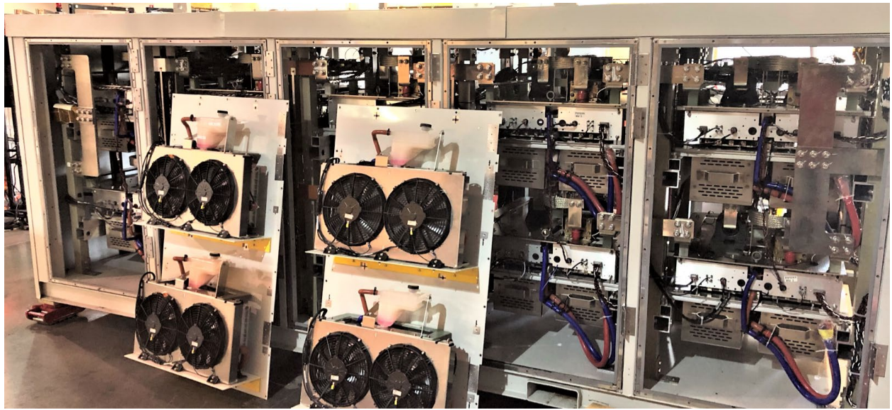
LCS side with panels removed
