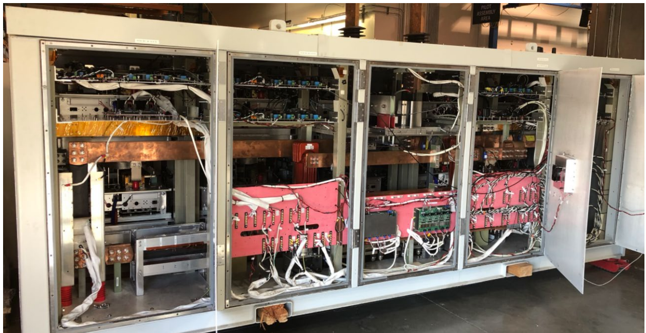
SV 10-3600i Main Internal Electromechanical systems
