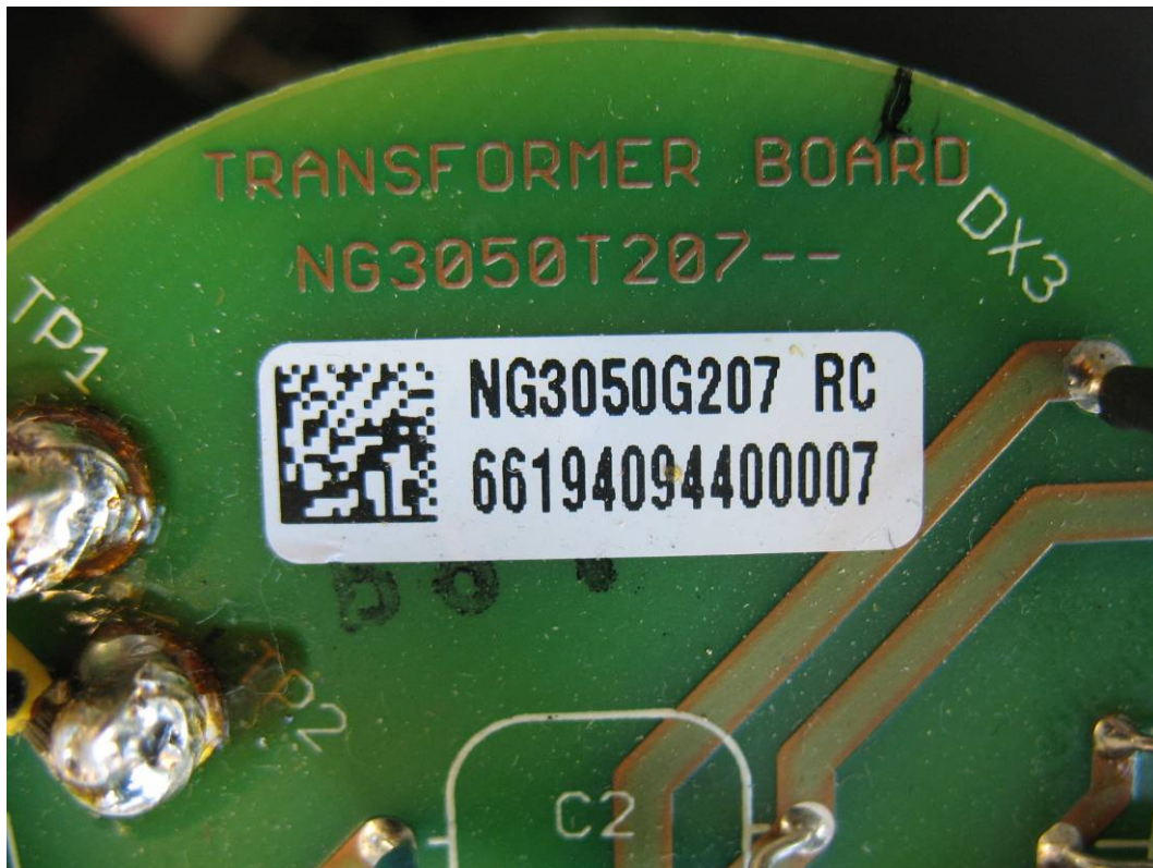
Photo No. 13: HV transformer, type label
