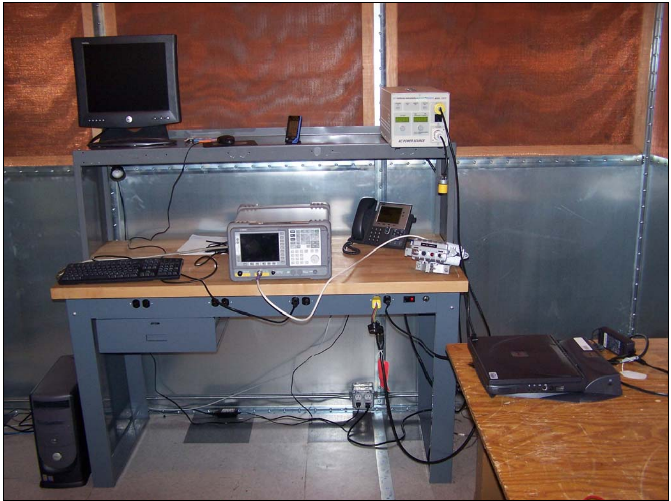
Photograph 5. Voltage Stability Test Setup
