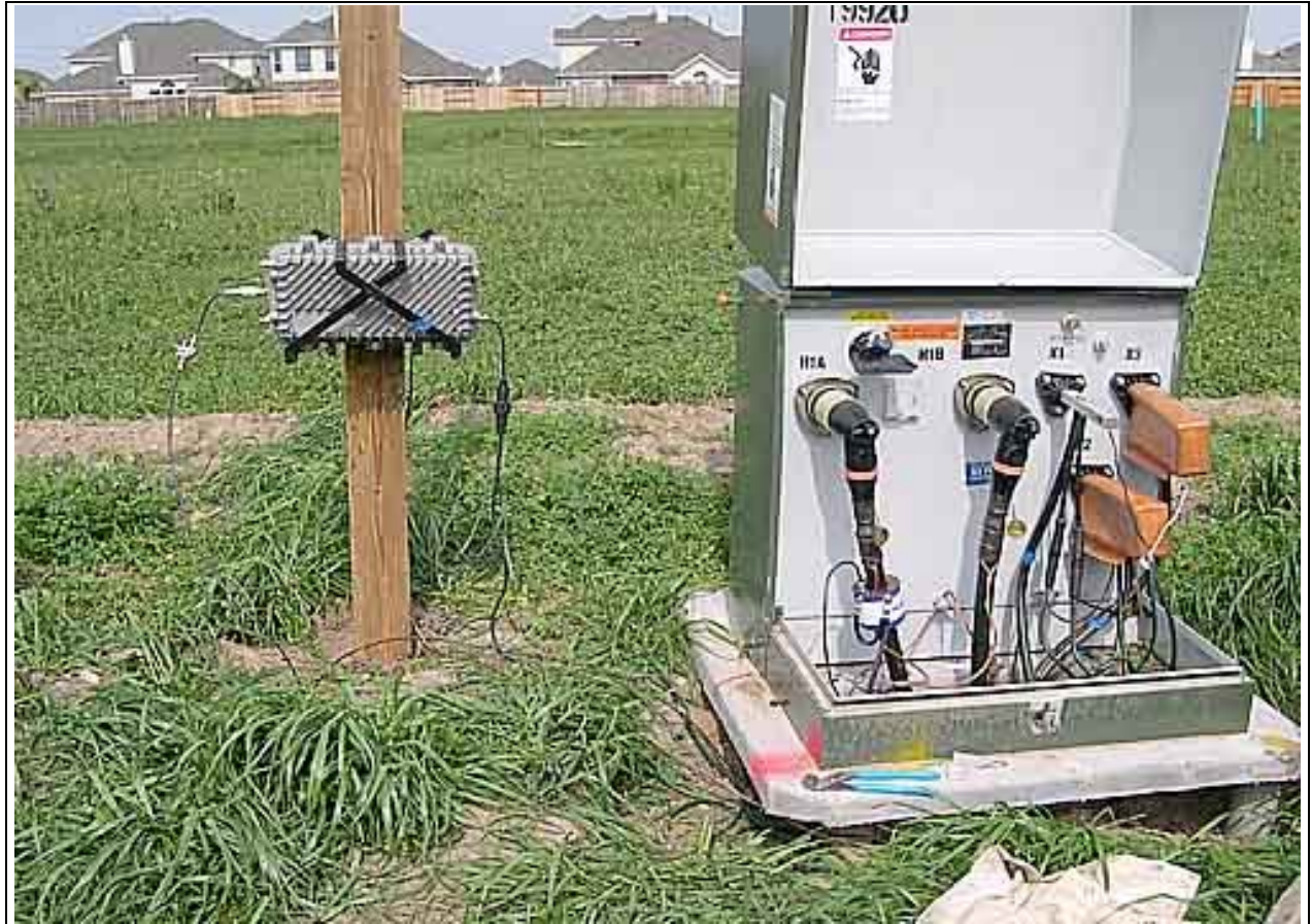
Unit and Coupler Installation with Transformer Door Open
