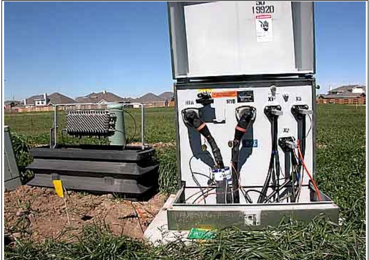
EUT and Coupler Installed
