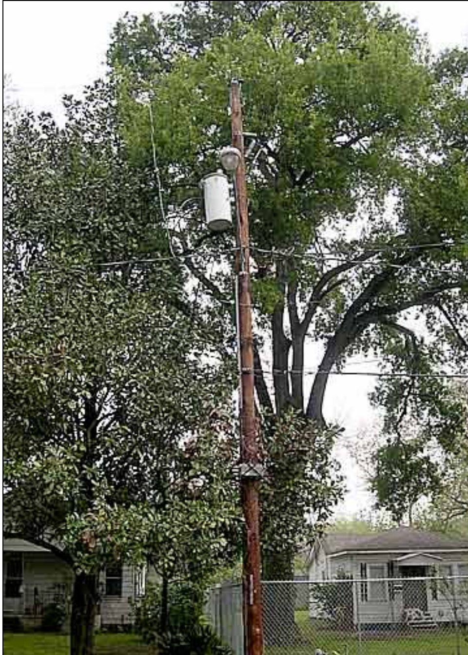
Unit on the Pole and Wire
