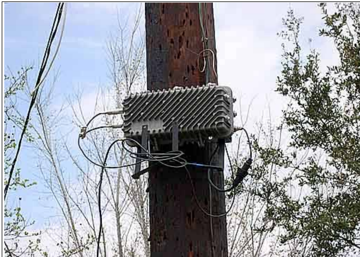
Corinex Medium Voltage Access Gateway/Regenerator
