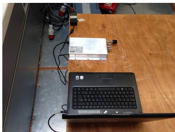
VPE Power supply Setup (Dummy Load)
