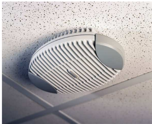
Figure 15 - Ceiling mounted nanoBTS
