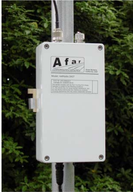
Figure 1.1. Pole Mounted Radio
