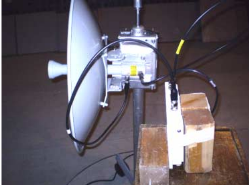
Photograph No.3 RADWIN 1000/2000 general view with external dish antenna
