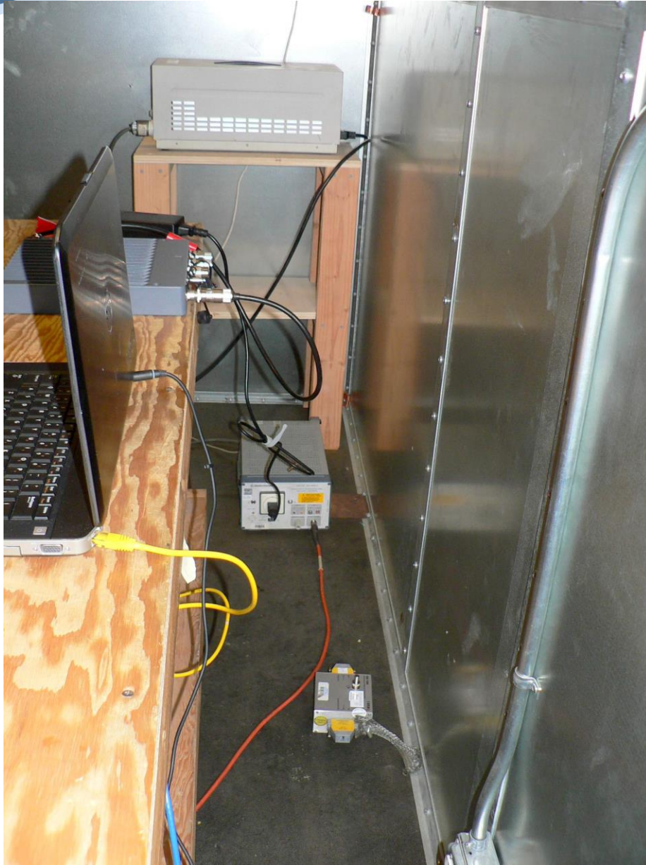
RDWN63 AC Wireline Side
