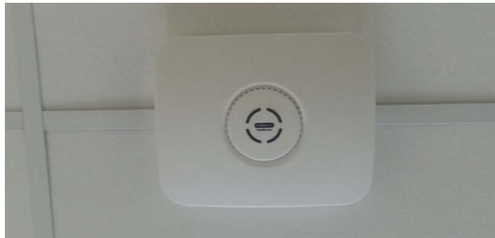
Figure 10: Controller mounted on a Floating Ceilings
