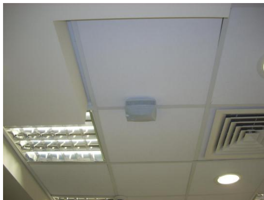
Figure 24: Exciter mounted on the ceiling
