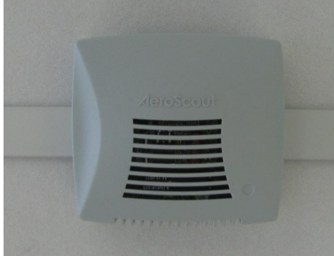
Figure 13: External Unit mounted on a false ceiling
