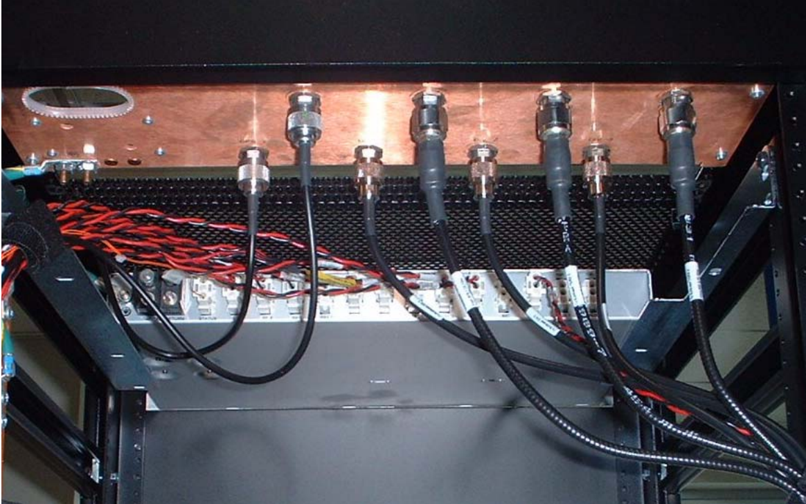
Figure 4.6 Top of Rack (TOR) Rear of the cabinet, Bulkhead, Cabling and Equipment
