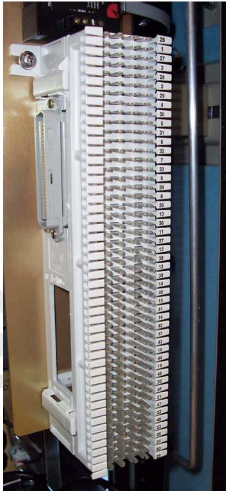
Figure 1.17 Punch Block Location within the MCSC system cabinet
