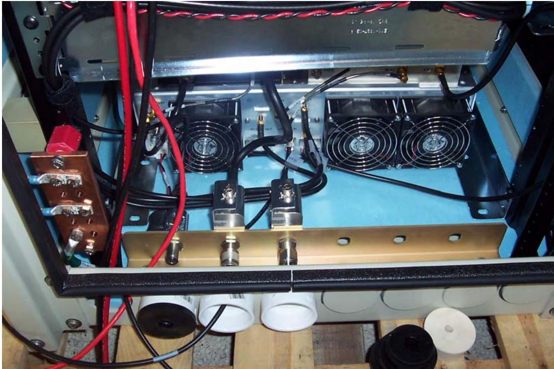
Figure 1.7 Top of Rack (TOR) Rear of the Cabinet, Bulkhead, Cabling and Equipment
