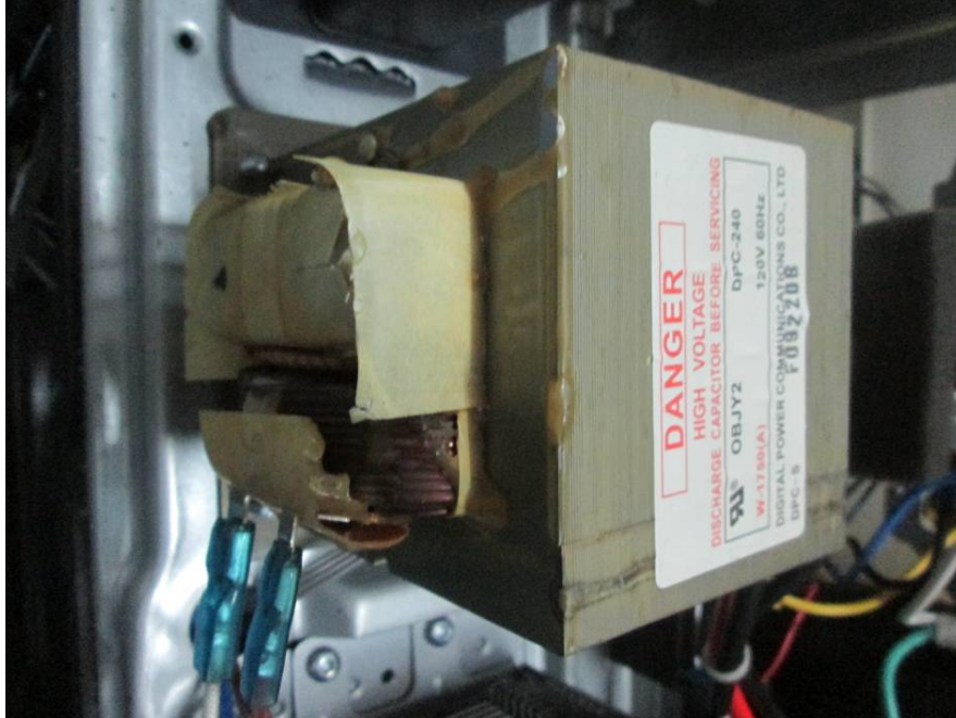
EUT – High Voltage Capacitor View
