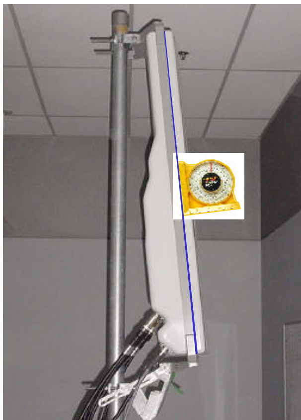
Figure 32: Measuring Antenna Downtilt
