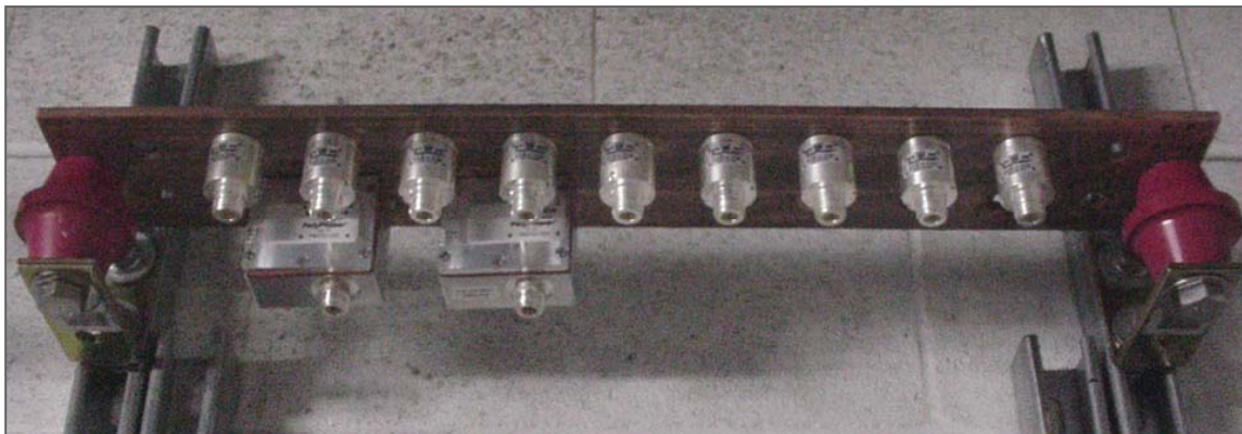
Figure 10: Surge Protectors in Buss Bar
