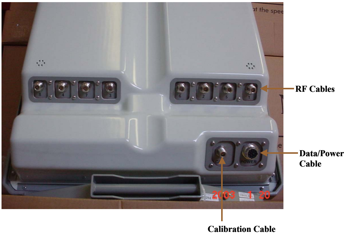
Figure 16: Panel Cable Routing
