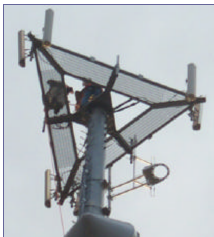
Figure 44: Secured Omni Antenna Mount
