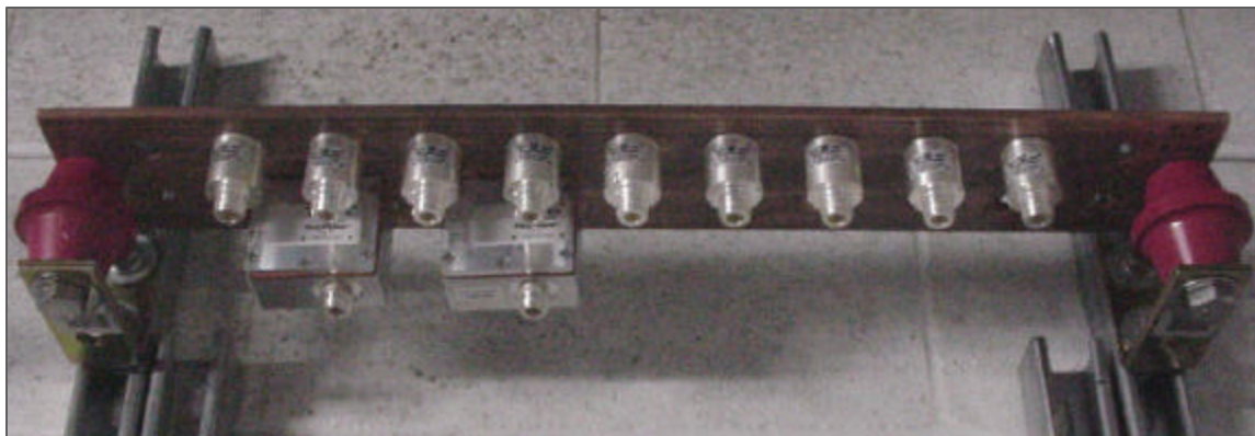
Figure 12: Surge Protectors in Buss Bar
