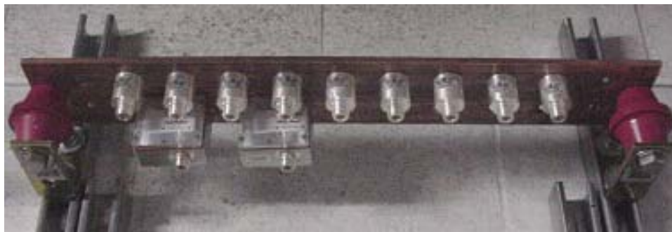
Figure 12: Surge Protectors in Buss Bar (Non-TTA system)
