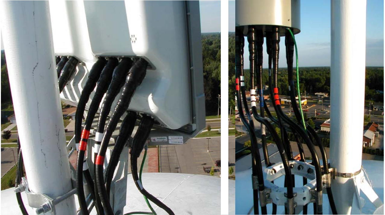
Figure 37: Weatherizing RFS Connectors Cables
