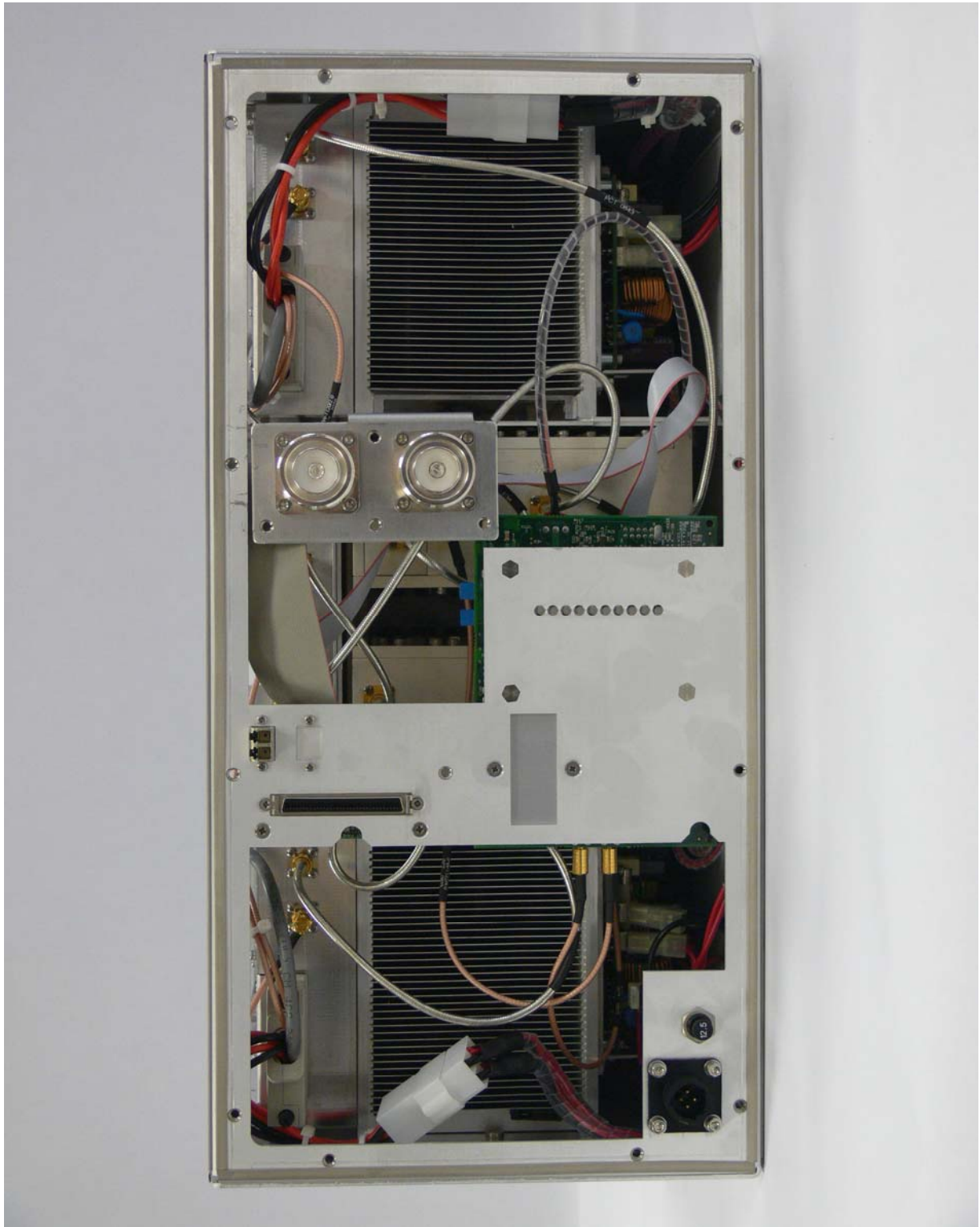
Figure 1: Radio Shelf – Front Panel Removed
