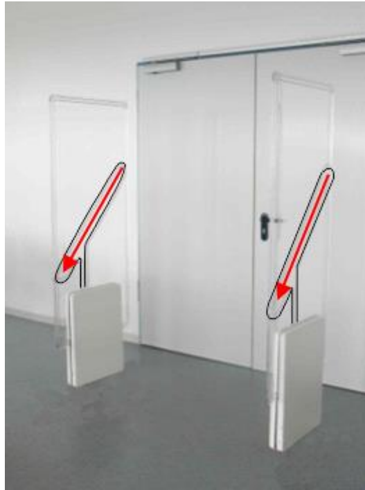
Figure 17: Direction of antenna conductor in front of Library door
