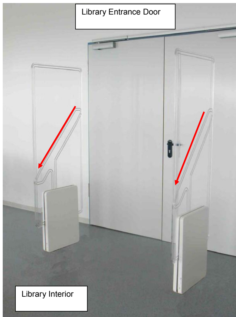
Fig. 12: Direction of antenna conductor in front of Library door
