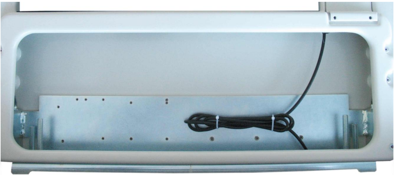
Fig. 12 Unused coaxial cables are tied in antenna Type B/BL
