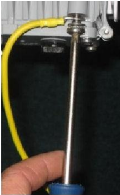
Figure 27 – attaching ground cable to AirSynergy
