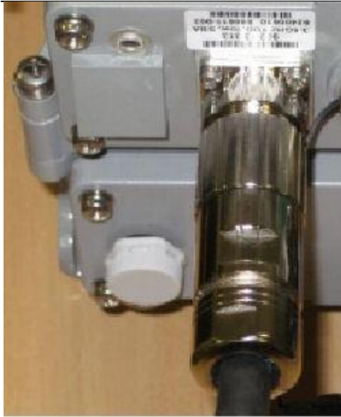
Figure 31 - attaching power cable to AirSynergy
