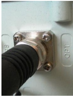
Figure 49 - Fiber-optic cable connected
