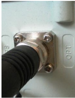
Figure 56 - Fiber-optic cable connected
