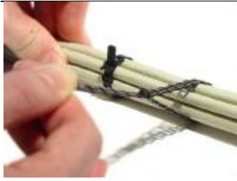
Figure 51 – Secure fiber-optic cable, use excess tie
