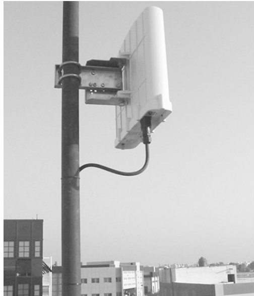
Figure 4-1: Typical BSR Installation
