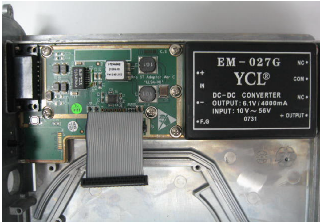
Photograph No.2 "ProST 698-746M Ext" power supply close view
