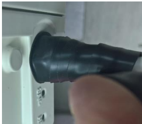
Figure 12: Weather-proof the CRTV RF Connection
