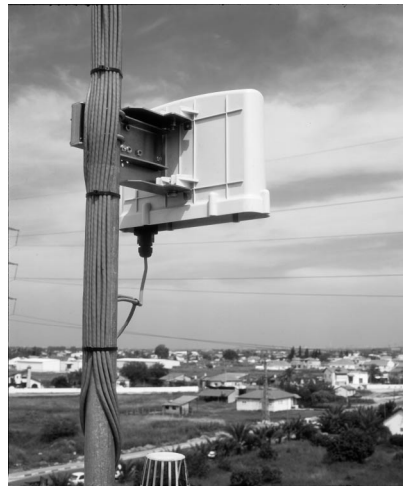
Figure 8-3: Typical SPR mounted outdoors on a pole
