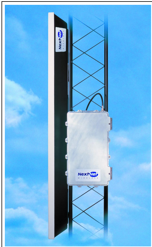
Figure 1.1 Base station mounted on tower with antenna connection
