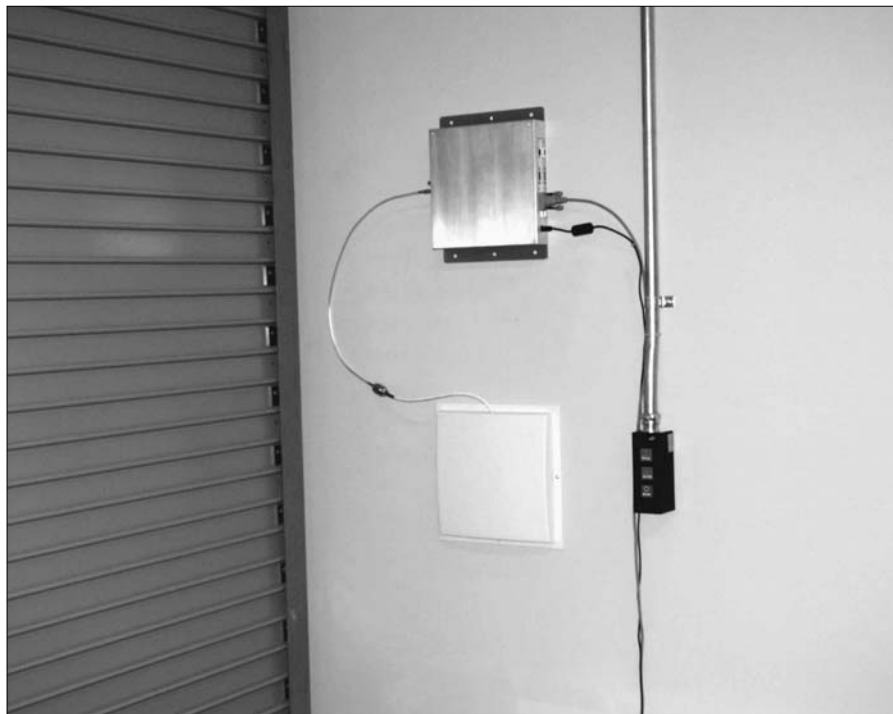
Nanoscanner system configured for a single-antenna portal application. Shown here at a loading dock.
