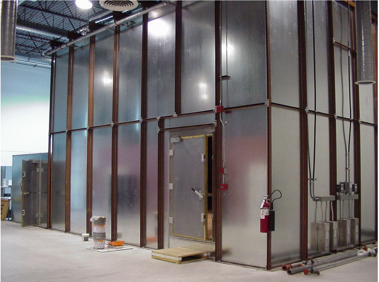
Article 10 - 3m Semi-anechoic chamber, Exterior view
