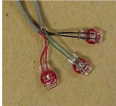
Figure 41 – Three Colored Wires Properly Connected
