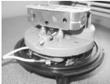
Figure 5: Connecting the module power leads to the meter power bus bars
