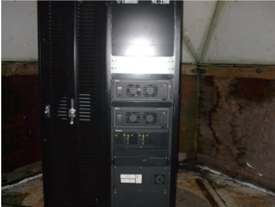
Emissions Test Setup Front View
