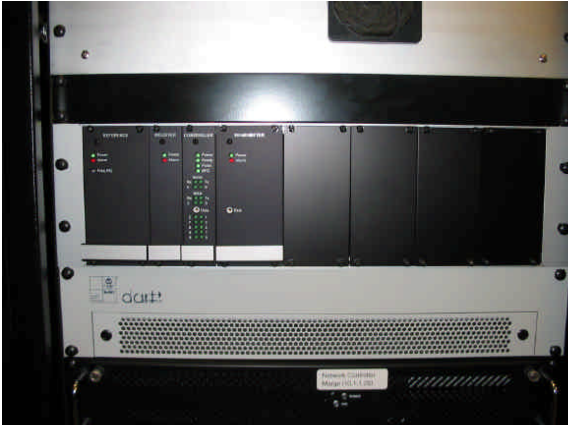
TUNet NC-2200 Network Controller Close up of RF/Control shelf.
