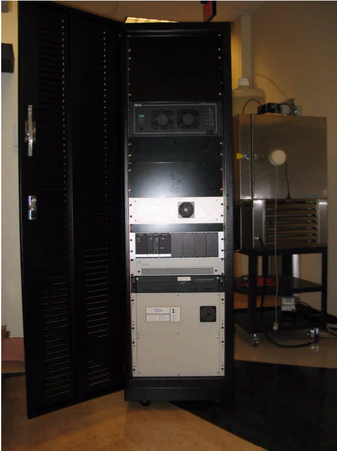
TUNet NC-2200 Network Controller Front view, front cabinet door open.
