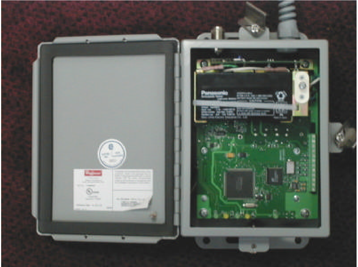
Internal View of Meter
