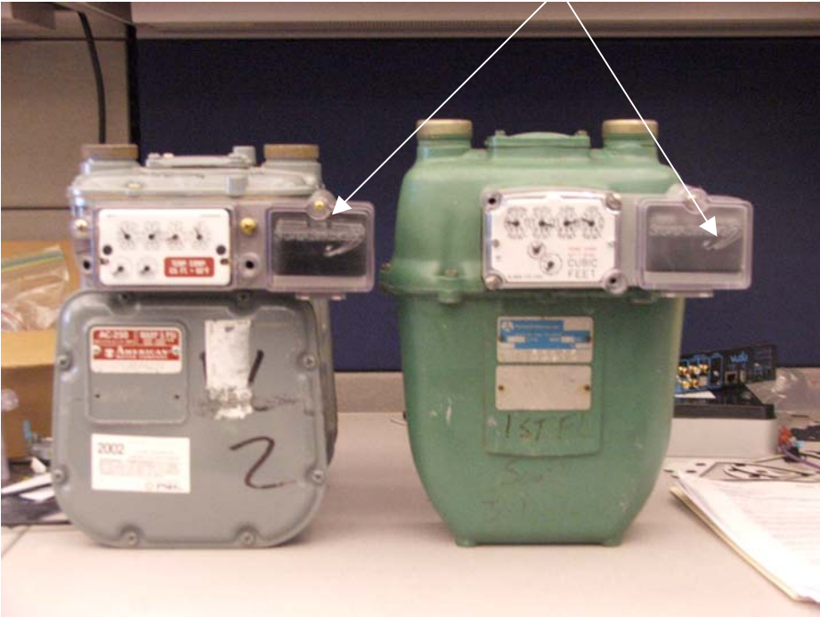
Plastic holder with radio module mounted on gas meters
