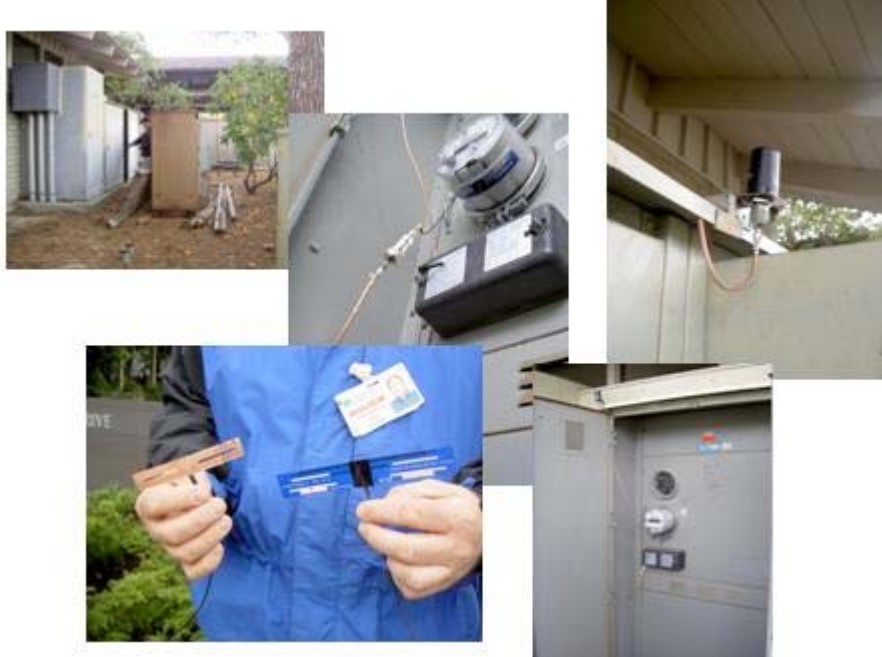
Figure 2. These photos of the MPACK Proof-of-Concept Test (10 Davis St., Belmont, CA, December 2009) show a typical metal enclosure for a commercial & industrial meter, two prototype MPACK coupling antennas, and a “salt shaker” style tamper-resistant antenna mounted temporarily at the top of the metal enclosure. The final product must, of course, be designed to be permanently and durably attached to the meter, the cables must be anchored to the meter panel and dressed neatly, and the antenna for metal enclosures like this is most likely to be a low-profile “hockey puck” style antenna bolted through the top of the enclosure and sealed with a gasket and adhesive, and connectors must be sealed against moisture.
