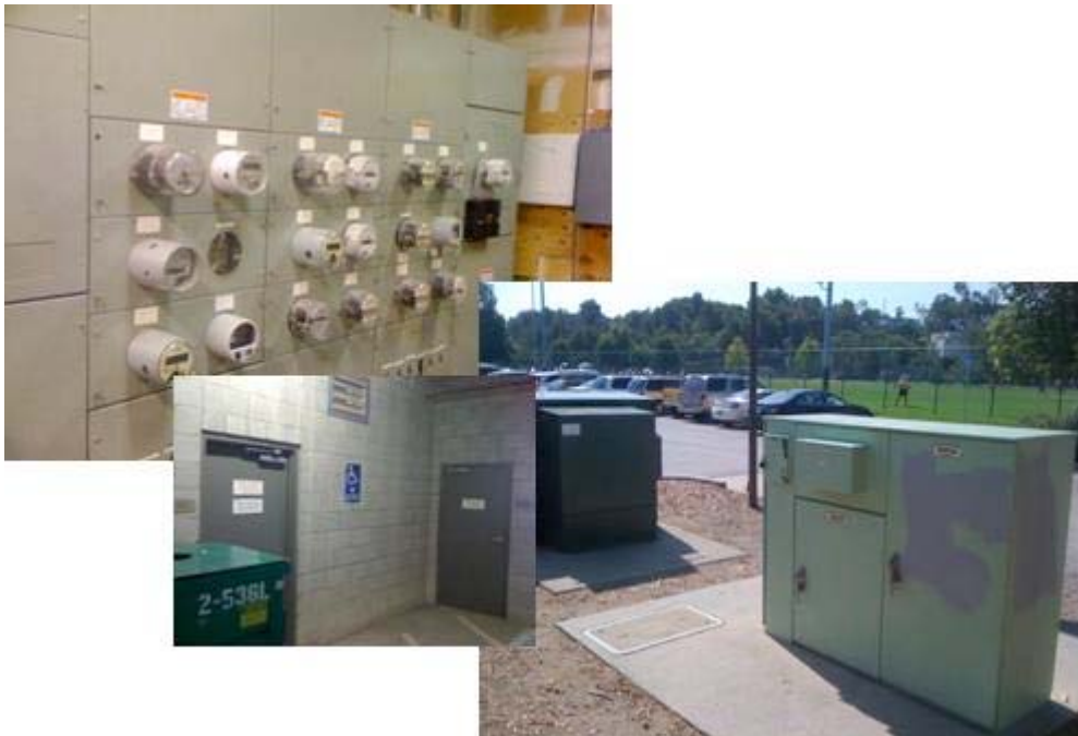
Figure 1. Meters in meter rooms and metal enclosures require external antennas.
