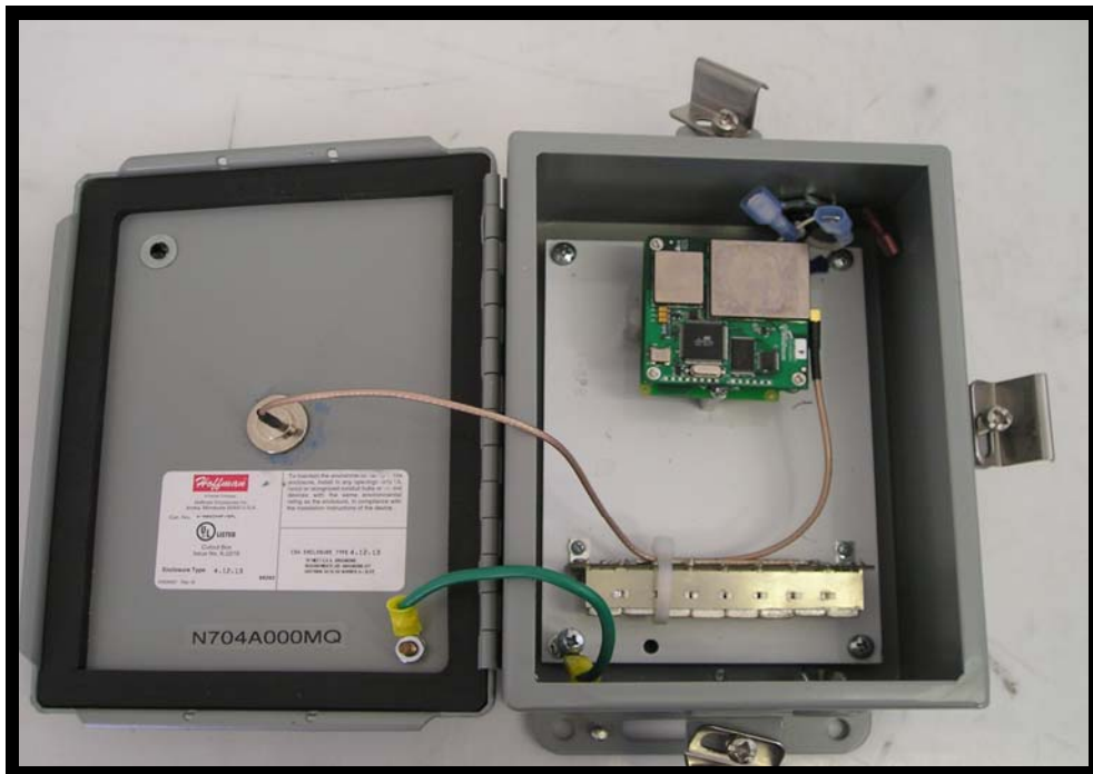
Figure 42: EUT Internal View1
