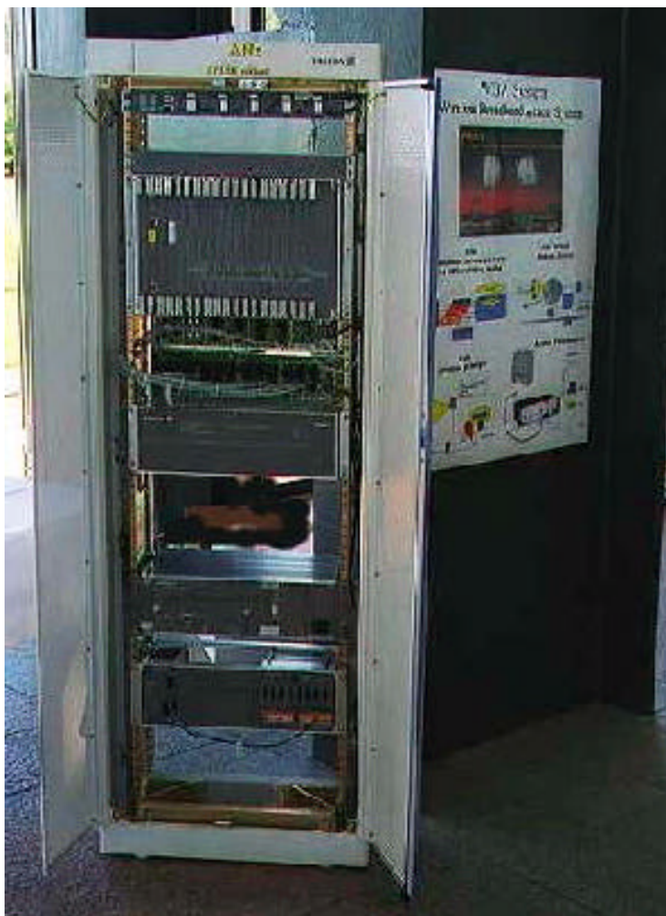
Figure 17. Example of indoor cabinet.
