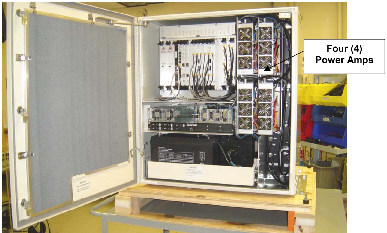
Figure 7-8 Power Amplifiers installed in RAN
