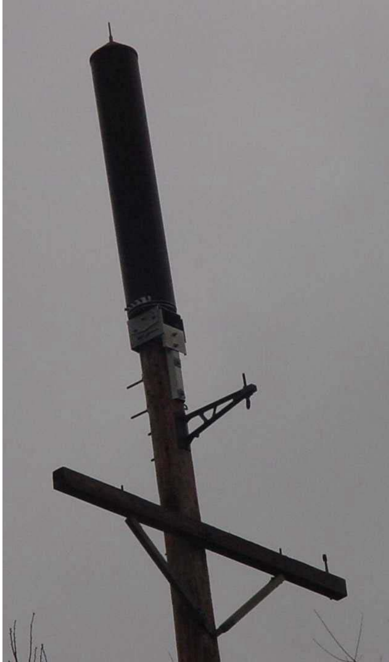
Figure 6-7 RAN Antenna Mounted on Pole
