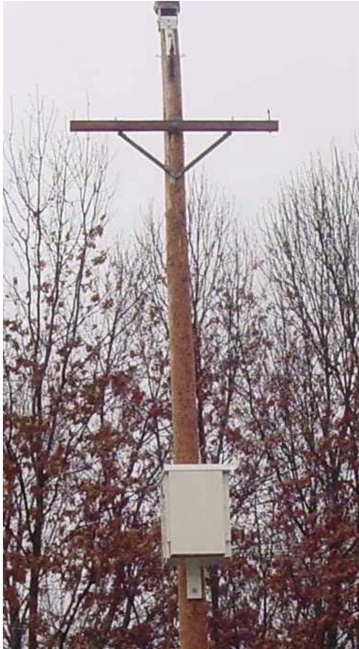
Figure 6-8 RAN Enclosure Mounted on Pole
