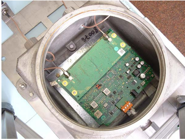
4070 IO Ex Top Removed Close up 1
